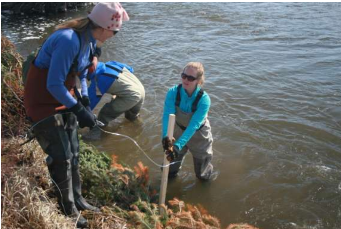
Teton Valley TU and Teton Regional Land Trust personnel work on stream-bank stabilization on Fox Creek
