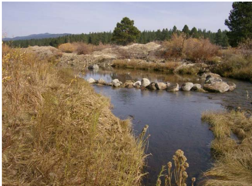
Photograph 2. Initial construction of a downstream facing “V” designed to direct water down a side channel on the right bank.
